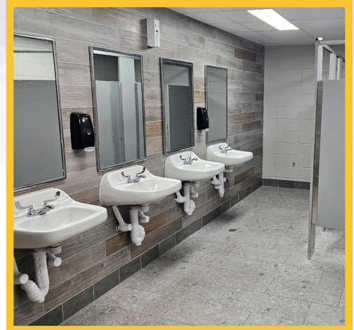
Restroom Refresh: Restroom facilities throughout the middle and high school saw worn fixtures replaced, as well as new flooring and paint installed.
