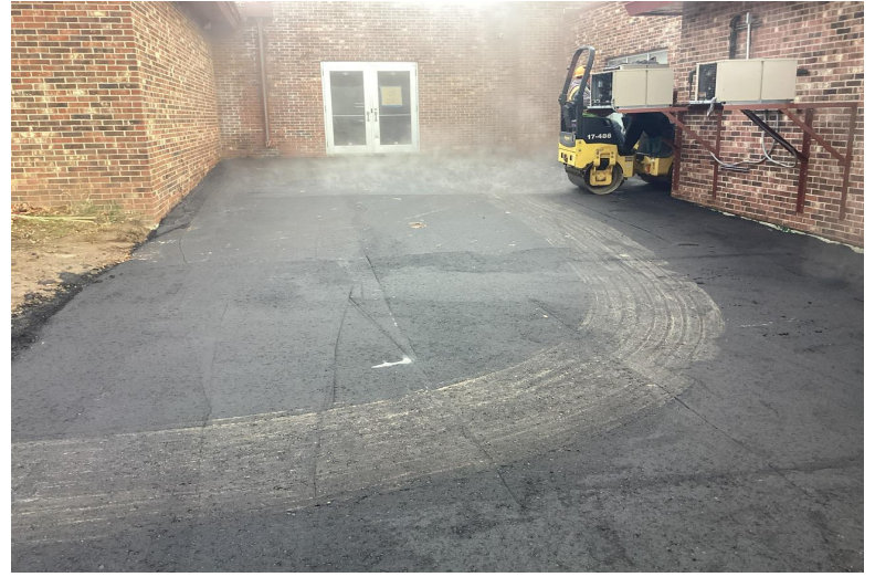
Binder course being installed for asphalt pavement at south parking lot/drive lanes
