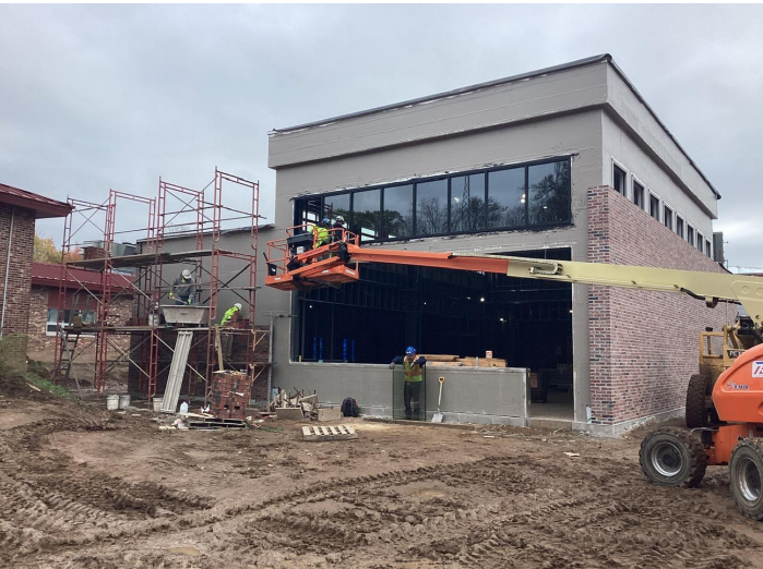
Exterior sheathing and vapor barrier and clerestory windows complete at Media Center
